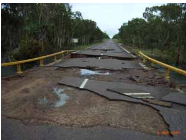
A washout and fairly major damage at the West Alligator River.
