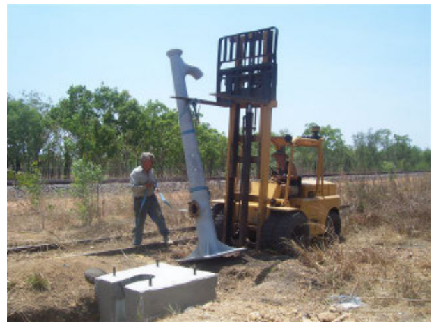
Alf and Trevor lining up the column to the south of the station.
